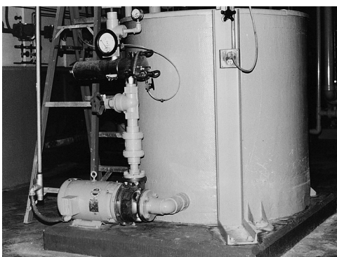
Reverse osmosis, Ósmosis invertida
