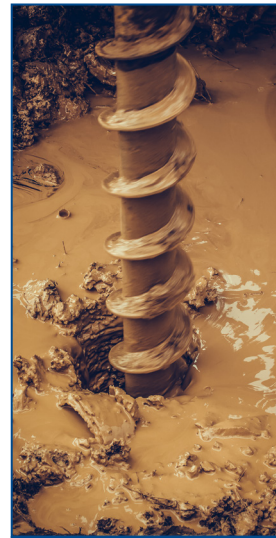
DRILLING MUD TRANSFER
